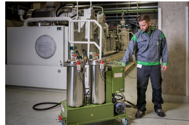
By-pass oil filtration
